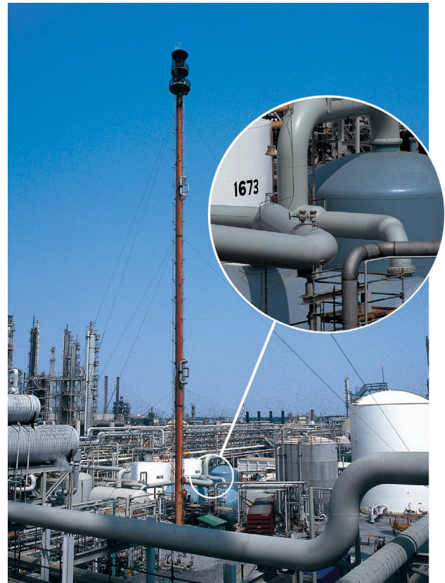
DigitalFlow GF868 field installation on a typical flare system. Insert shows transducers installed on the flare header that leads to the flare stack.
